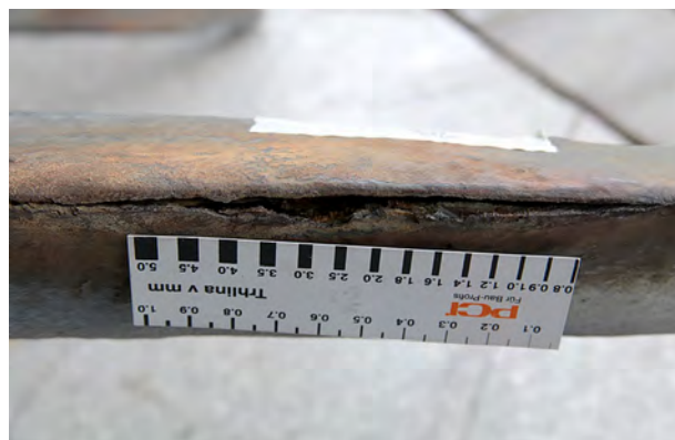
Obr. 3. Prasklina v celé tloušťce laminátu Fig. 3. Crack in the whole thickness of the laminate
